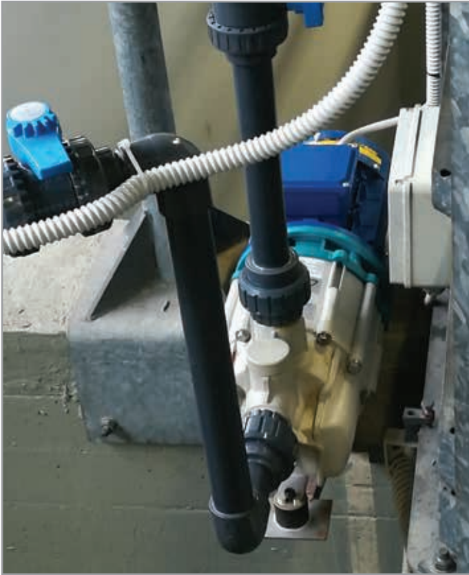
ITALY. Precious metal plant - RHINO (TMA G2) pump for wastewater transfer.
