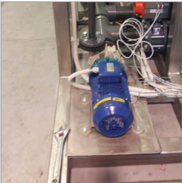
ITALY. Desalination plant ROUTE pumps for transferring Sodium Hypochlorite for seawater electrochlorination processes.
