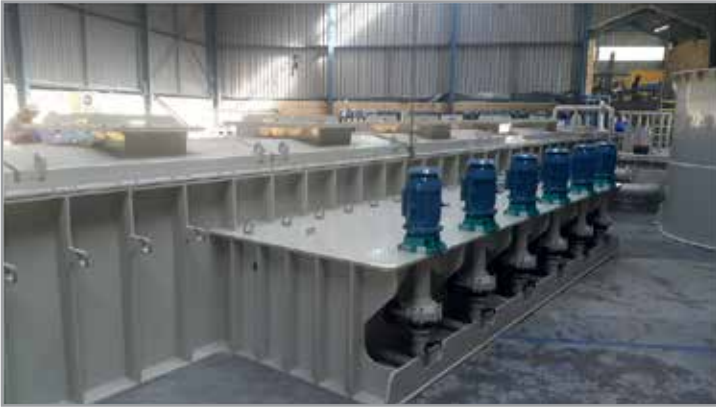
SOUTH AFRICA. Wire pickling plant EQUIPRO (HME) for transferring strong acids from a tank to another.
