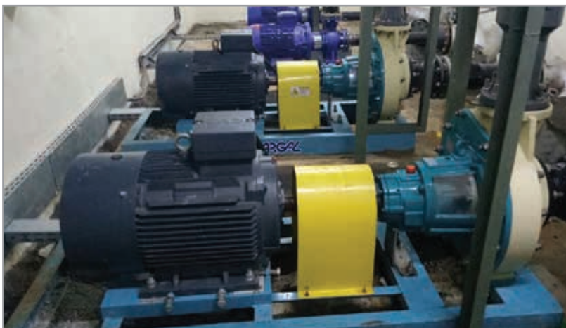
INDONESIA. Safari park for supplying the main pool with seawater
