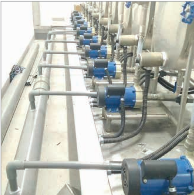
CHINA. ASP oil recovery plant - BASIS pumps for recirculation of percolates.
