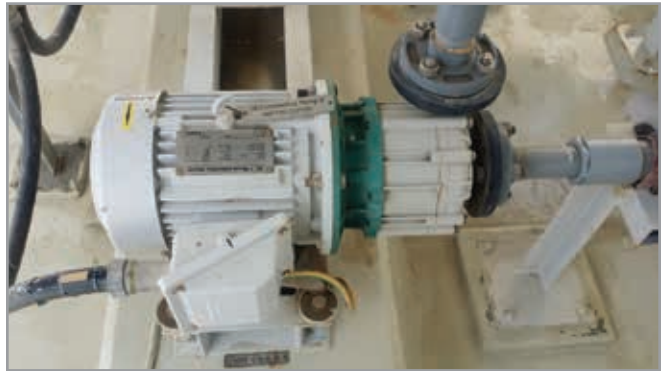
KUWAIT. Power plant - ROUTE pump for unloading NaOH.
