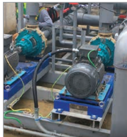
THAILAND. Electrochlorination plant for the dosing of Sodium Hypochlorite and seawater.
