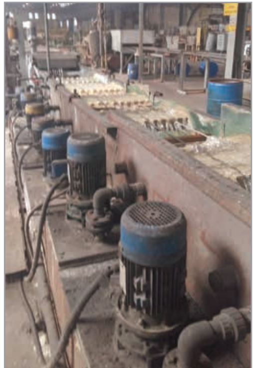
ITALY. Pickling plant K2 (KGK) for transferring concentrated hydrochloric acid.
