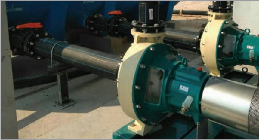
THAILAND. Aquaculture plant - for supplying the seawater tanks
