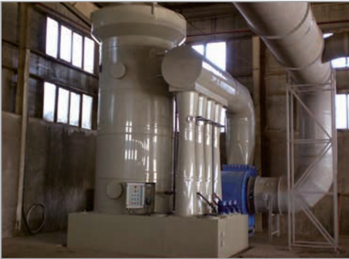
ITALY. Fume scrubber plant K2 (KGK) & EQUIPRO (KME) for conveying cleaning solution for taking off toxic gases from liquids.
