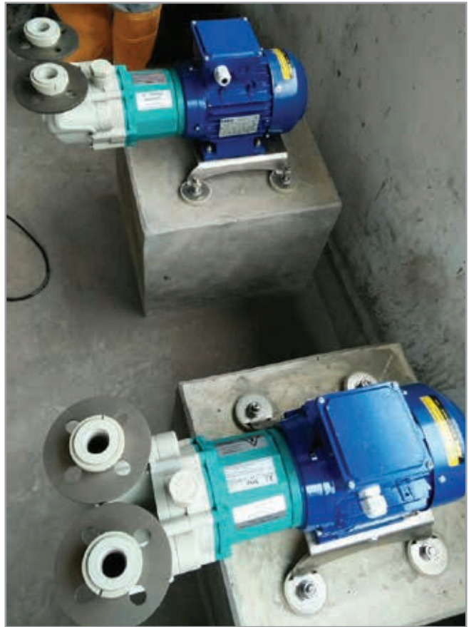
INDONESIA. Chemical plant - ELK (TMA G1) pumps for transferring water charged with toxic agents.
