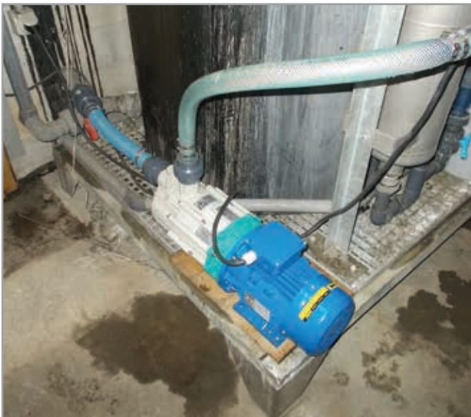
SWITZERLAND. Garage - RHINO (TMA G2) pumps for unloading wastewater containing cleaning products, oils and acids.
