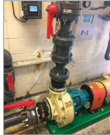
USA. Aquarium - for transferring seawater
